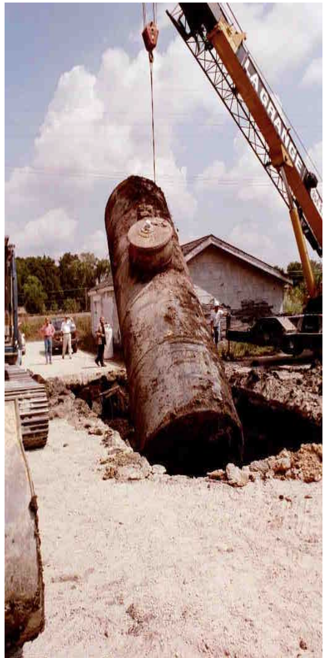
Tank removal is often the first step in the cleanup of an underground tank release.
