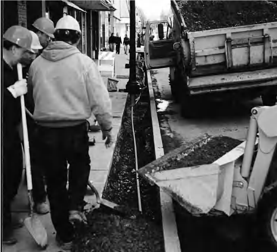
Fig. 27. Structural soils in continuous planters, under sidewalks, and under asphalt allow tree roots to grow while supporting the weight of cement and asphalt. The actual planting pit is filled with fertile soil.
