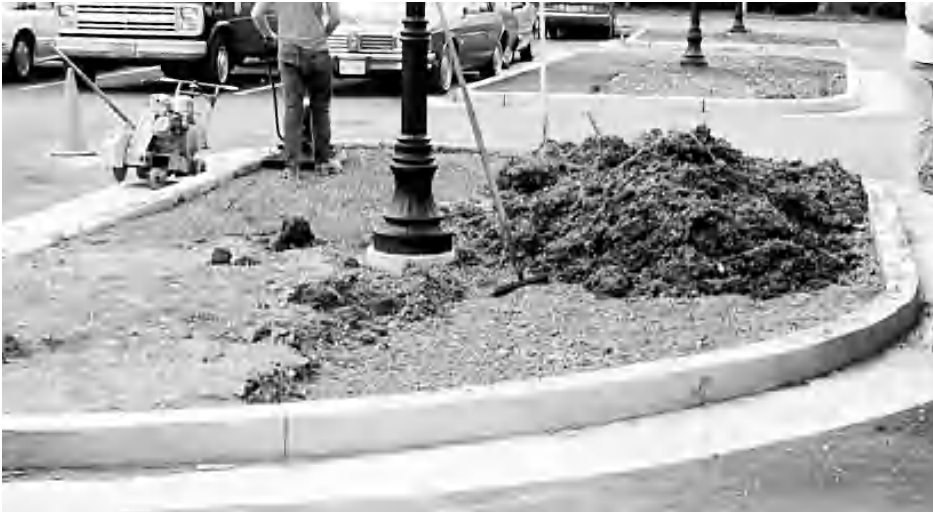
Fig. 32. Placing a thin amount of soil over compacted gravel or clay does not allow for good plant growth. The parking lot planter should be well drained and filled with a minimum of 4 feet of fertile topsoil.
